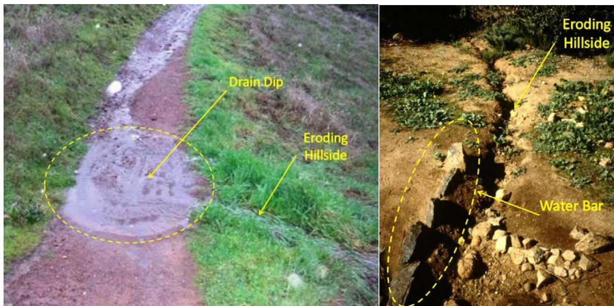
Photo 26.2 - Drain Dip (left) and Water Bar (right) Discharge Eroding Hillslope
