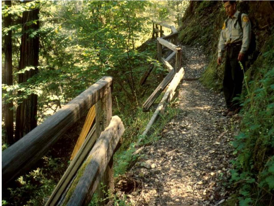
Photo 26.15 - Railing Damaged by Falling Limbs
