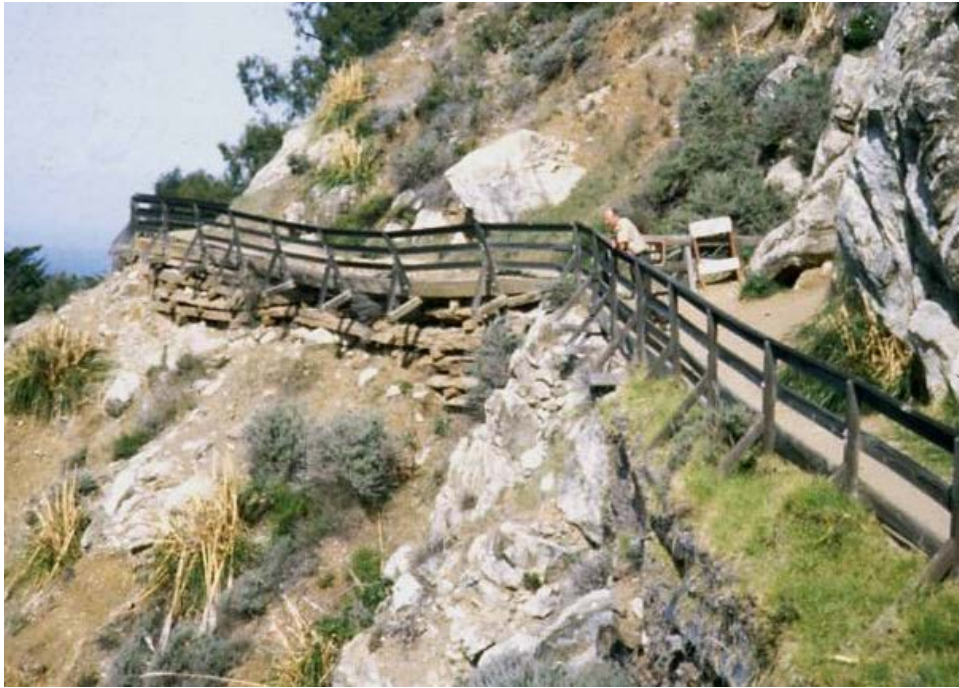
Photo 26.17 - Retaining Wall Needing Replacement
