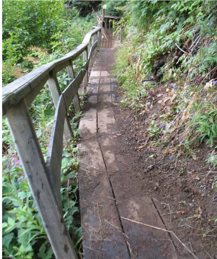
Photo 26.14 - Railing in Need of Replacement
