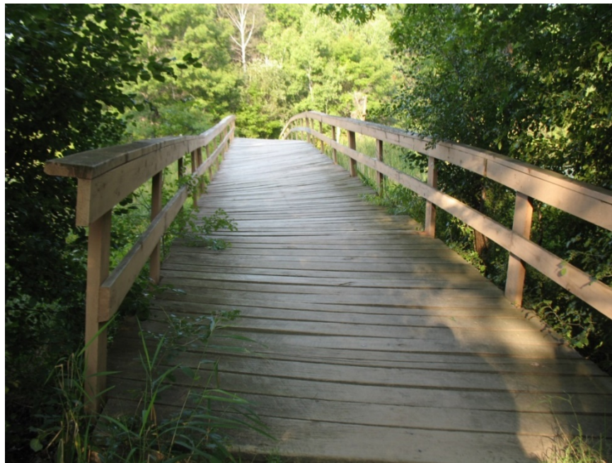
Photo 26.10 - Boardwalk in Need of Replacement
