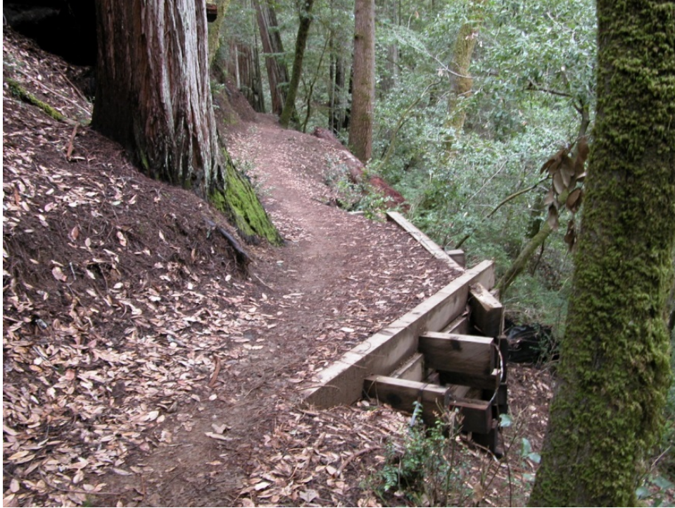
Photo 26.16 - Retaining Wall Higher than Trail Tread
