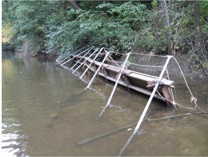
Photo 26.7 – Washed out Pipe Bridge
