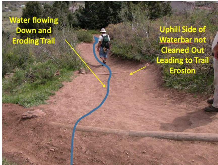
Photo 26.3 - Unmaintained Water Bar
