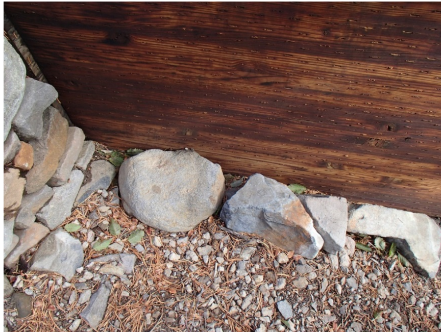
Photo 26.6 - Bridge Stringer with No Air gap
